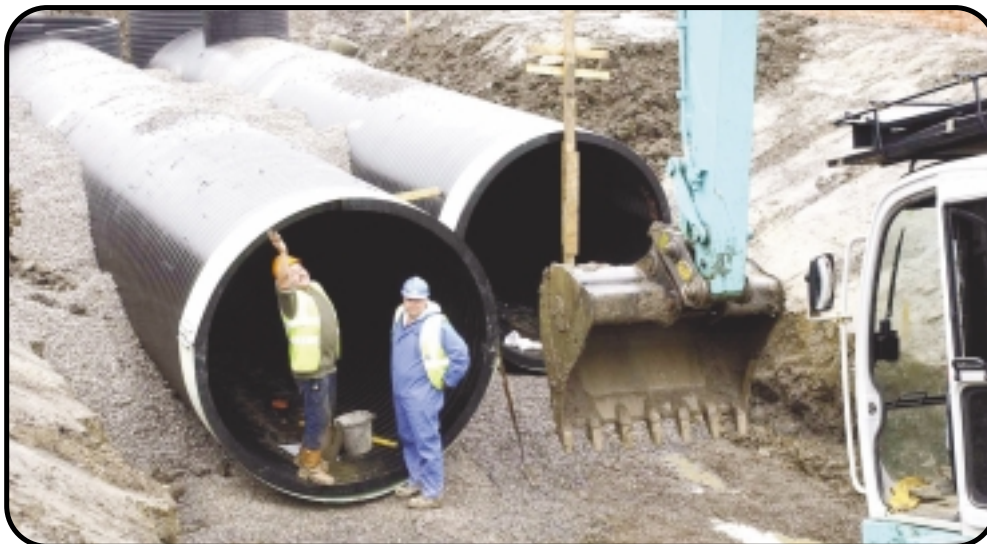
Construction on target thanks to the innovative use of WEHOLITE pipes supplied by ASSET International Ltd to the Welsh Water Capital Alliance. Pictures courtesy of the Swansea Evening Post
